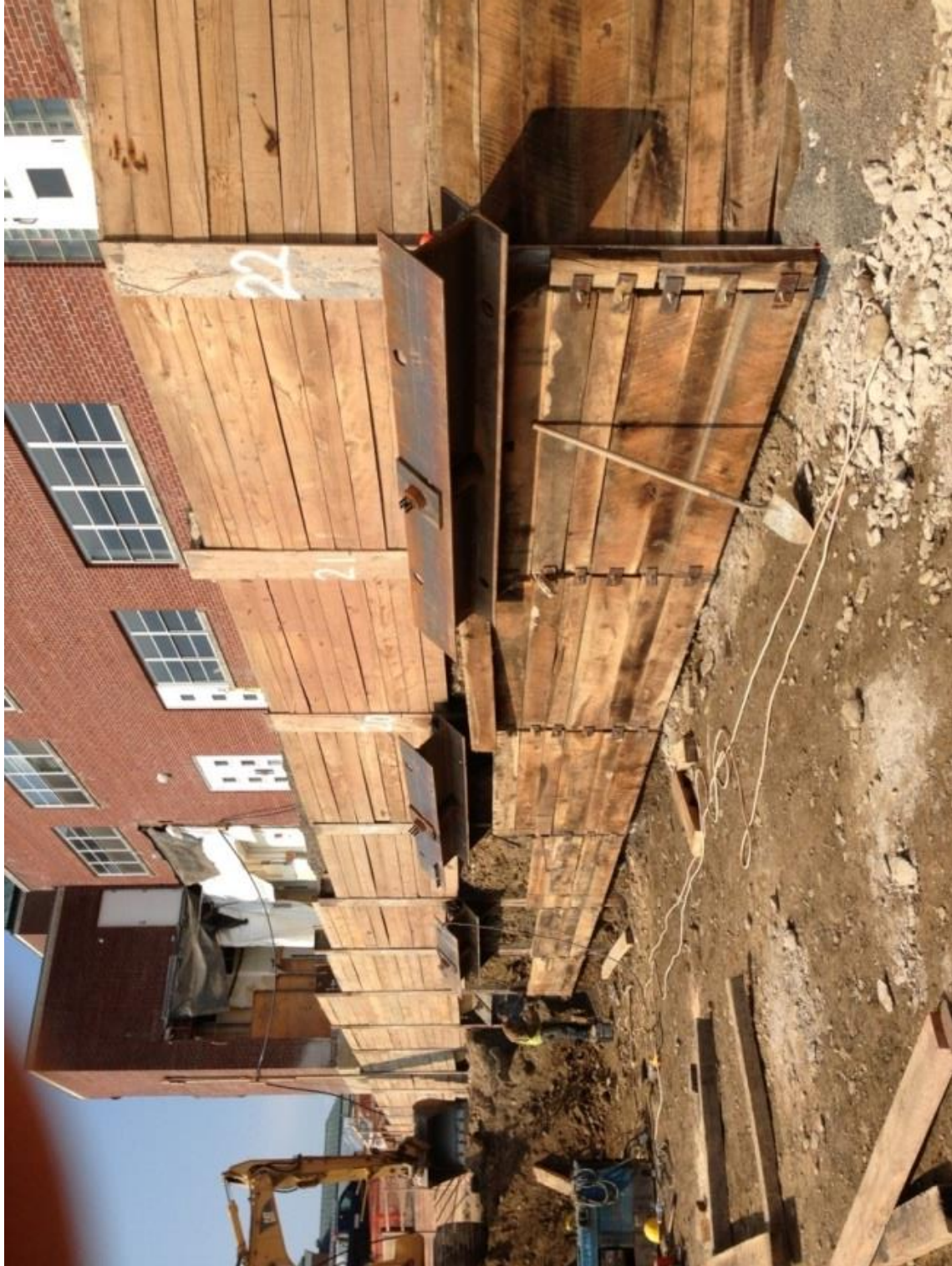
Figure 6-10. Picture of Hartwick College retaining wall with the building that was underpinned
